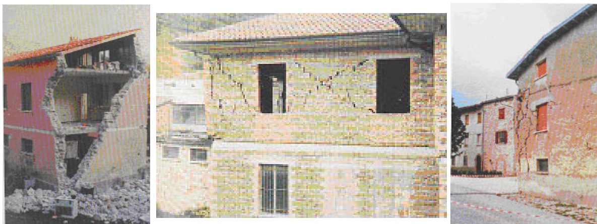
Figure 3 – Examples of cracks in buildings
